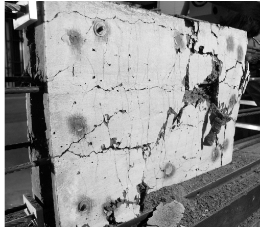
b) specimen with rebars and fibers (applied tensile strain is 3.5 ‰)
